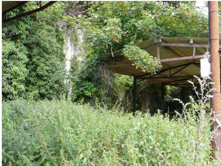
3. Third open shed showing vegetated chalk face behind. Grid ref. TQ14820572. Direction NW.
