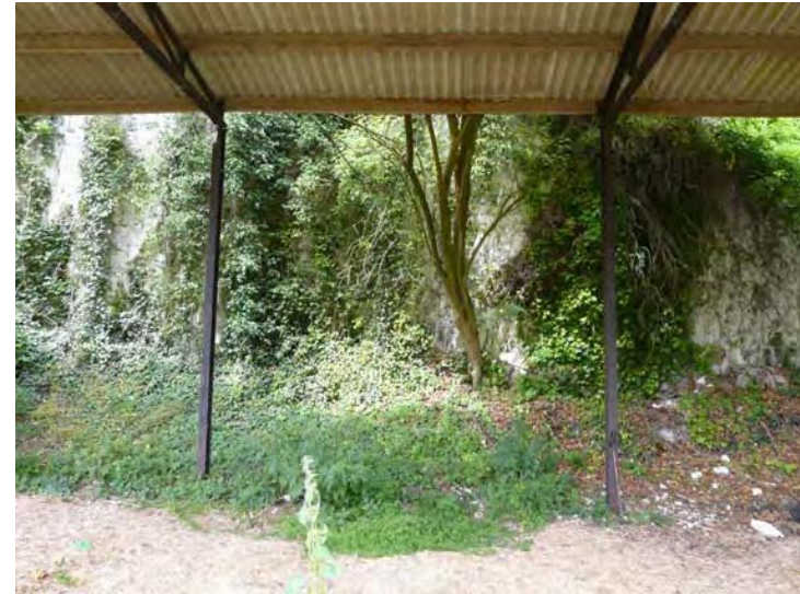
4. Vegetated chalk face at back of third open shed. Grid ref. TQ014820574. Direction west.
