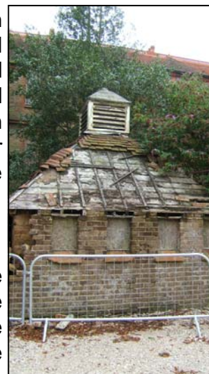
Fig. 24: Run down buildings
