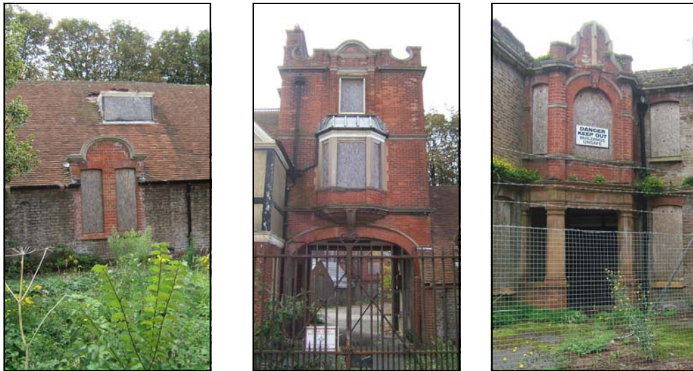
Figs. 5, 6, 7: Architectural details (from left): Dutch gable on entrance block, entrance arch on entrance block, entrance to refectory block
