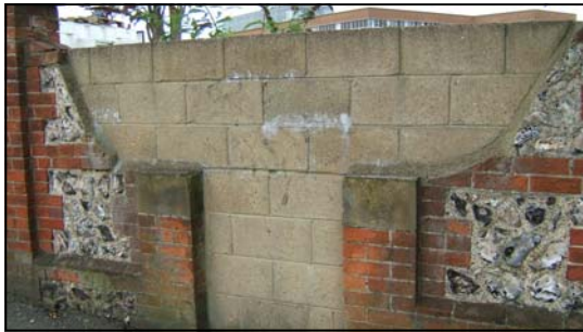
Fig. 26: Inappropriate filling of access point
