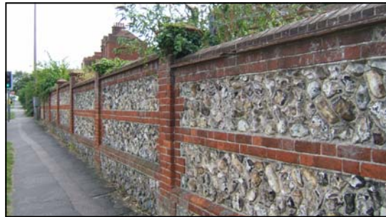
Fig. 21: Front boundary wall
